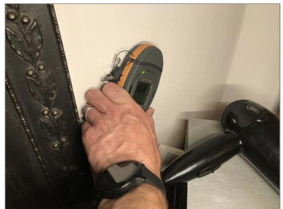
Photo - 83 Damp meter testing to bedroom fireplace.
