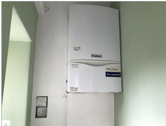
Photo - 110 Combination boiler.
