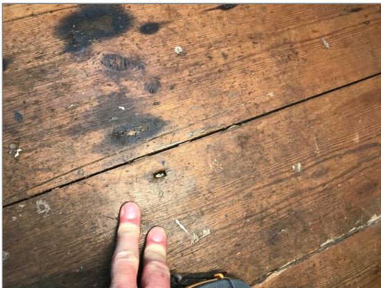
Photo - 76 Loose floorboard in entrance hallway.
