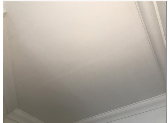
Photo - 33 Minor cracking to hallway ceiling.
