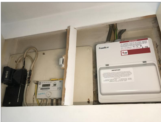
Photo - 102 Electricity meter and distribution board.
