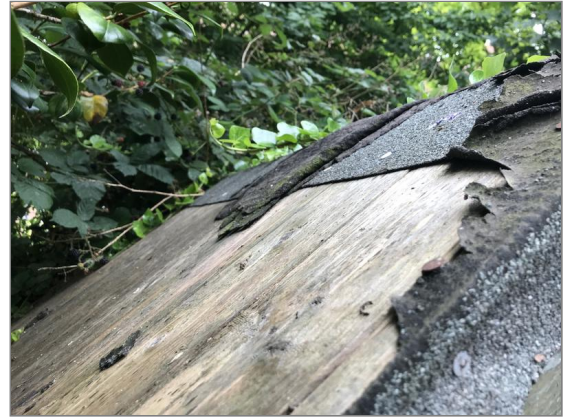
Photo - 125 Failed roof coverings to shed.
