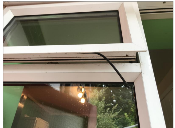
Photo - 17 Loose gasket to kitchen windows.
