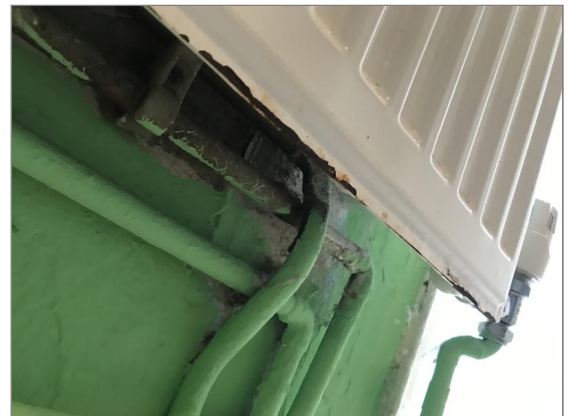
Photo - 109 Rust to kitchen radiator.
