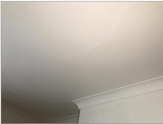
Photo - 34 Minor cracking to living room ceiling.
