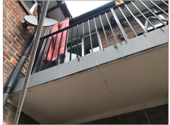
Photo - 30 Failure of decorations to walkway at rear of property.
