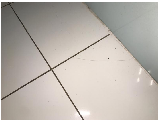
Photo - 72 Cracking to bathroom tiling.
