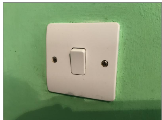
Photo - 105 Single plastic light switch in kitchen.
