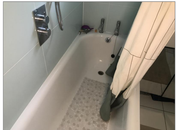
Photo - 99 Bathroom fittings.
