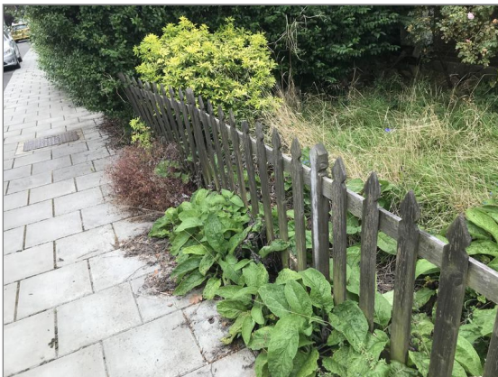
Photo - 120 Deflection of front garden fence.
