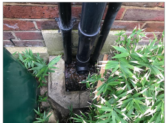
Photo - 10 Build up of debris in open gully.
