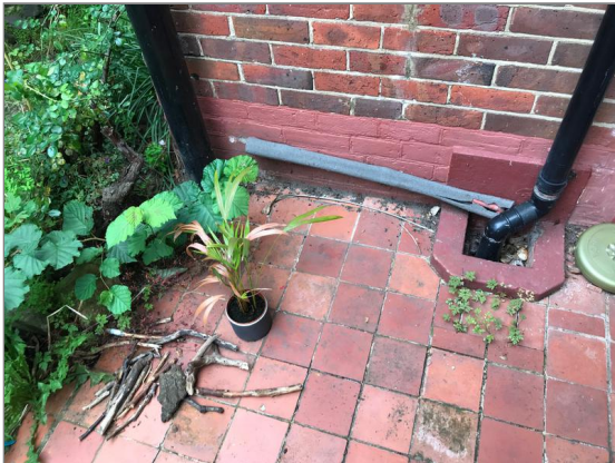
Photo - 116 Open gully at rear of property.
