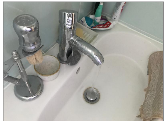
Photo - 113 Drop in hot water supply.
