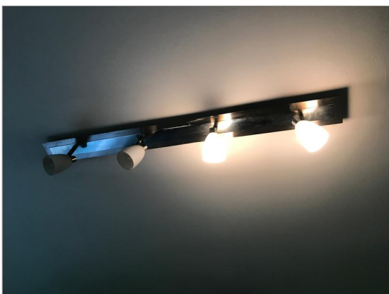
Photo - 104 Bulkhead light fitting in kitchen.
