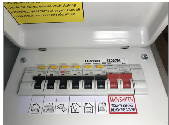
Photo - 103 Distribution board.
