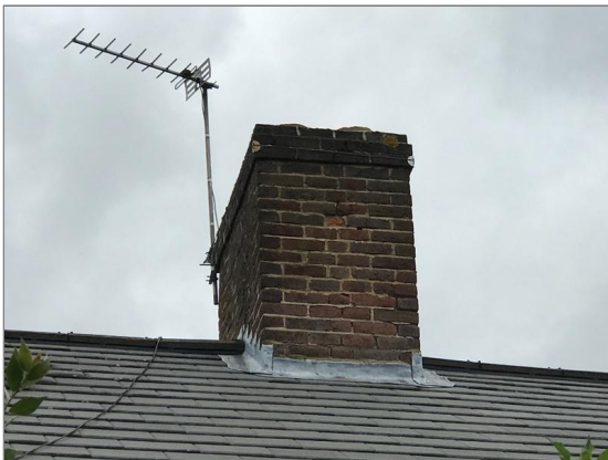
Photo - 6 Frost damage and failure of pointing to main chimney stack.
