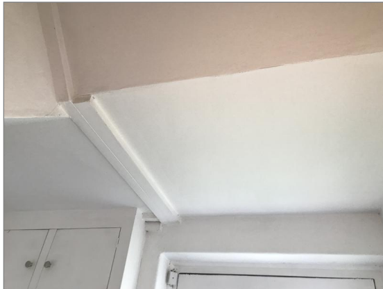
Photo - 32 Entrance hallway ceiling.
