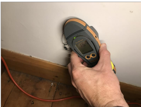
Photo - 51 Damp meter testing to bedroom walls.
