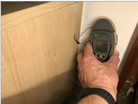
Photo - 80 Damp meter testing to front sitting room fireplace.
