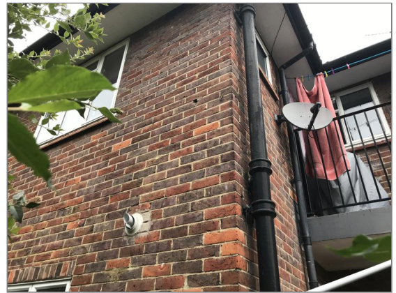
Photo - 15 Brickwork at rear of dwelling.
