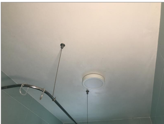
Photo - 38 Bathroom ceiling.
