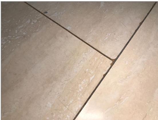
Photo - 70 Scuffing to kitchen floor.
