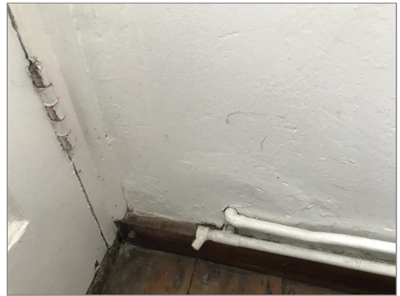
Photo - 42 Live area of plaster in entrance hallway.
