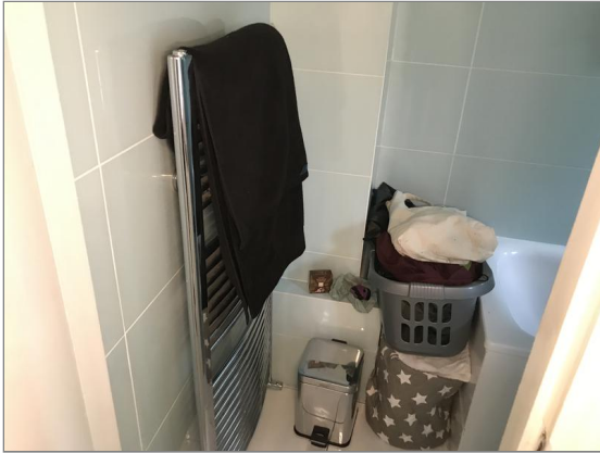
Photo - 84 Chimney breast enclosed in upon in bathroom.
