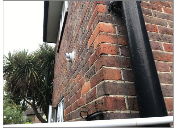
Photo - 85 Boiler flue penetrating side of property.
