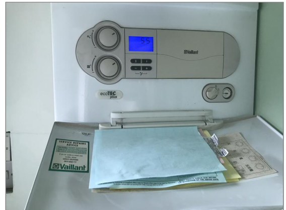
Photo - 111 Combination boiler panel.
