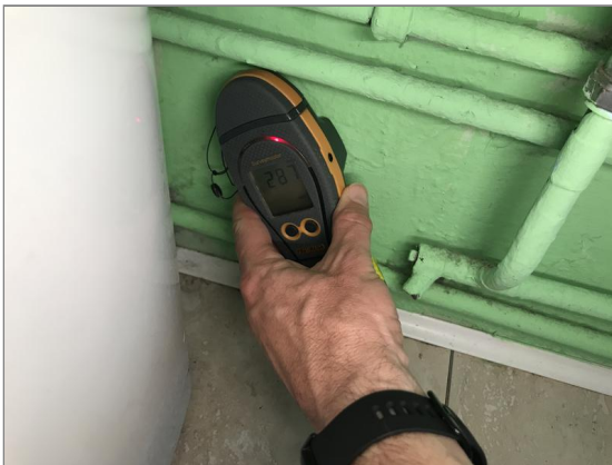
Photo - 55 Elevated damp meter readings to kitchen walls.
