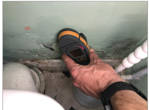
Photo - 66 Water penetration through WC walls.
