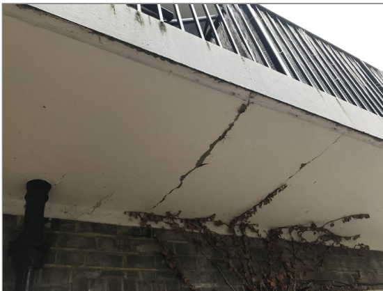
Photo - 31 Failure of decorations to walkway at rear of property.
