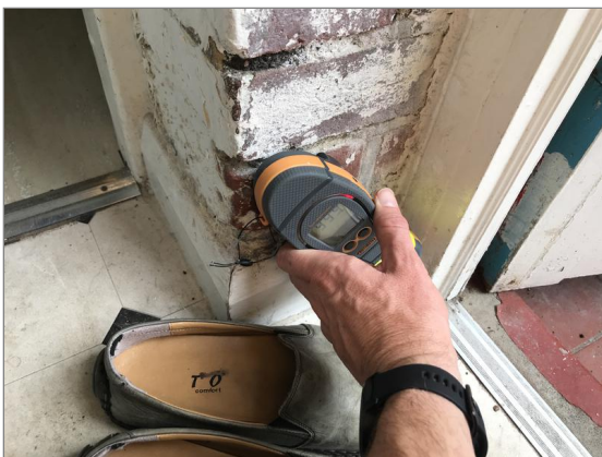
Photo - 63 Damp meter testing adjacent to rear door.
