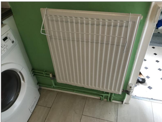
Photo - 108 Kitchen radiator.
