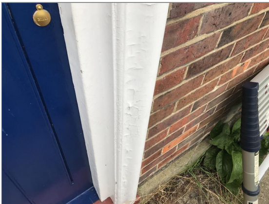
Photo - 25 Failure of decorations to door frame.
