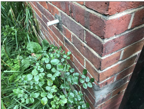
Photo - 67 Plant growth adjacent to area of water penetration.
