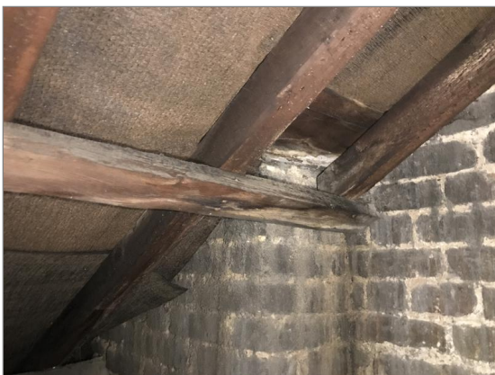
Photo - 78 Water damage to roof timbers in contact with chimney stack.
