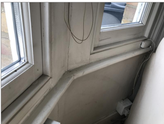
Photo - 55 Failure of internal decorations to living room window.
