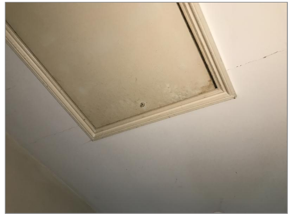
Photo - 83 Cracking to the landing ceiling.
