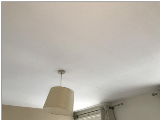
Photo - 80 Front bedroom ceiling.
