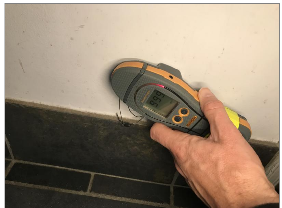
Photo - 104 Dampness to kitchen walls.
