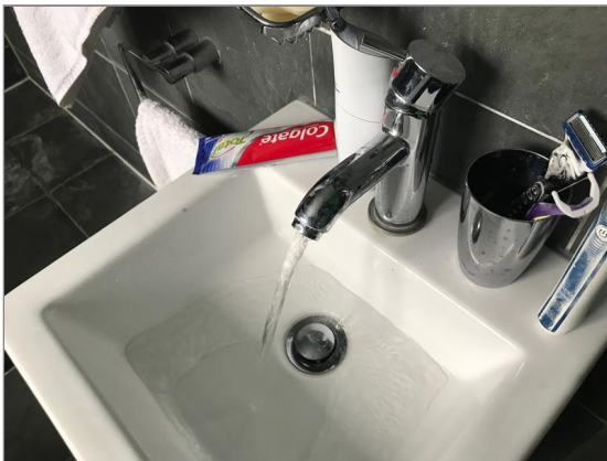
Photo - 175 Testing hot water supply.
