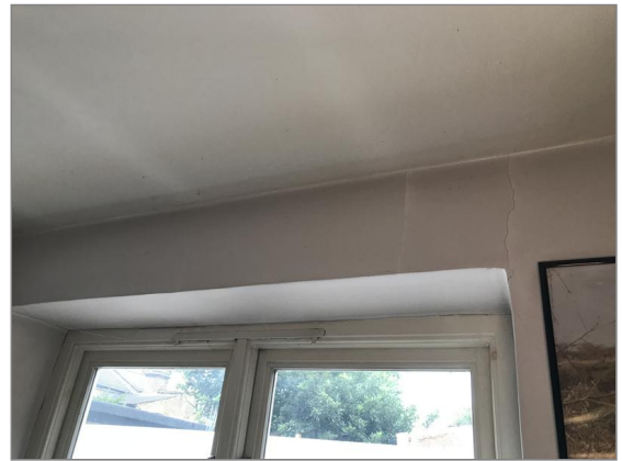
Photo - 100 Humidity damage to kitchen walls.
