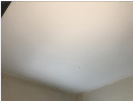
Photo - 84 Cracking to landing ceiling.
