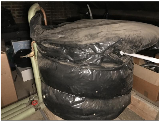
Photo - 167 Cold water tank in the loft.
