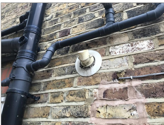
Photo - 139 Boiler flue.
