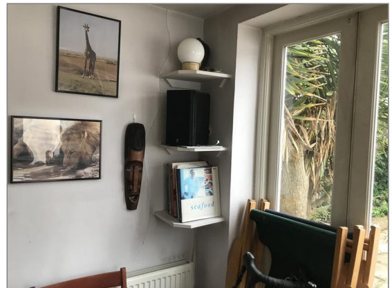
Photo - 98 Cracking to dining area walls.
