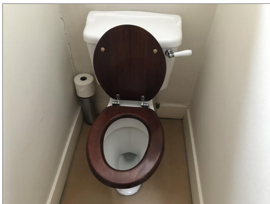
Photo - 156 WC fittings.
