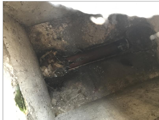
Photo - 177 Slight blockage to front garden inspection chamber.
