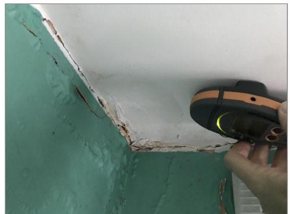
Photo - 87 Water penetration damage to bathroom ceiling.
