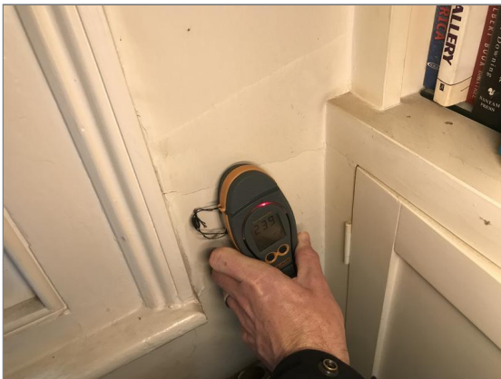
Photo - 113 Elevated damp meter readings to rear sitting room walls.
