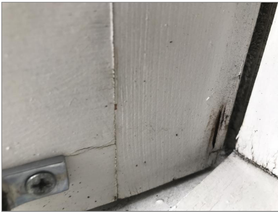
Photo - 51 Slight decay to landing window.
