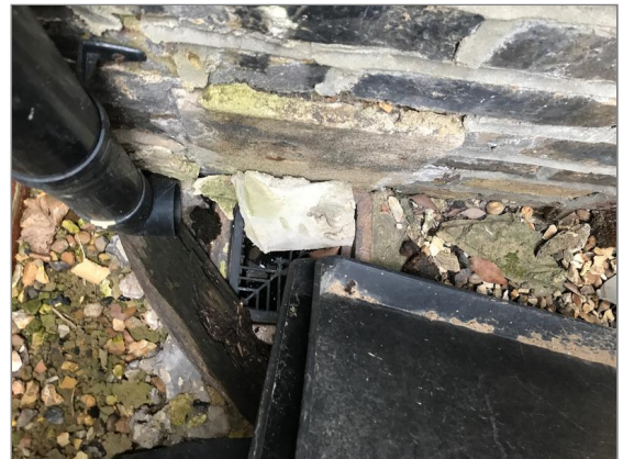
Photo - 25 Adjustment required to rainwater downpipe.
