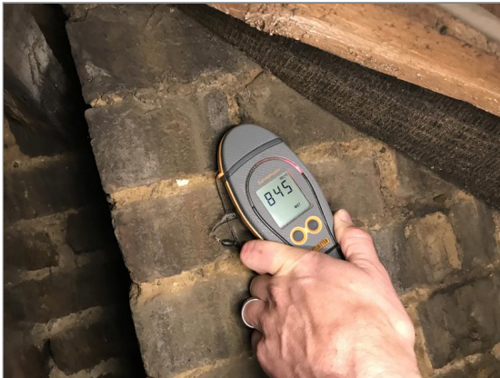
Photo - 76 Elevated damp meter readings to chimney stacks.
