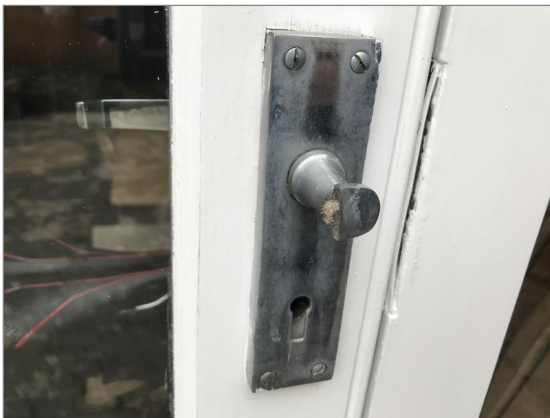
Photo - 66 Damage to folding door handle.
