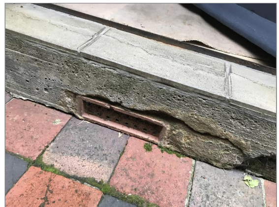
Photo - 134 Sub floor vent in contact with ground.
