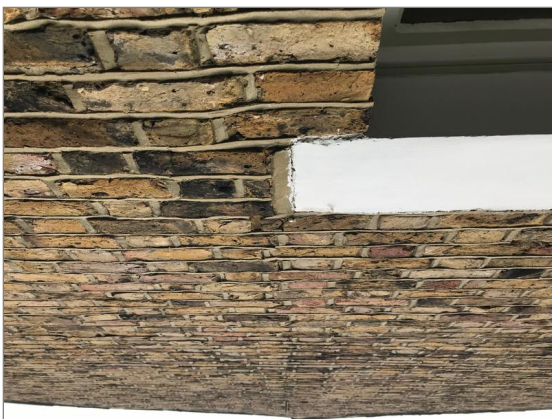
Photo - 36 Cracking above front door.
