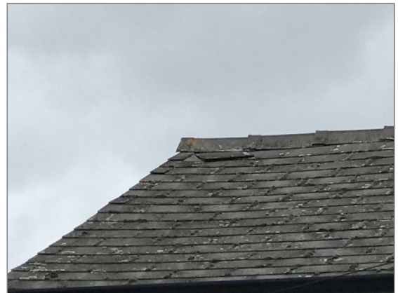
Photo - 12 Loose slate to front pitched roof.
