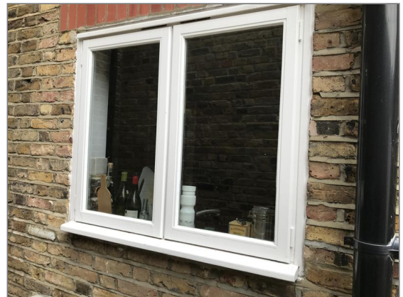
Photo - 60 Kitchen window.
