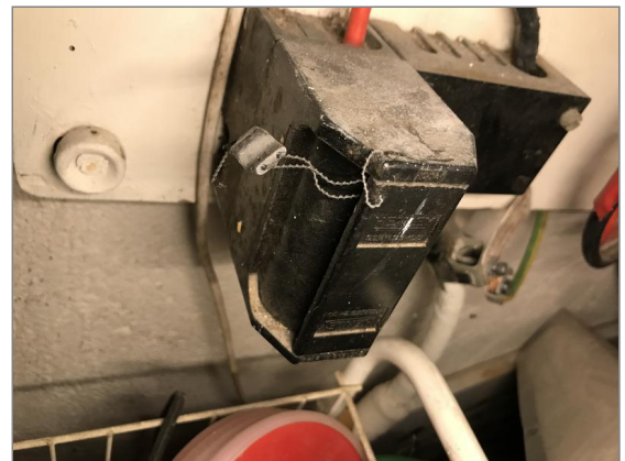
Photo - 162 Incoming main.
