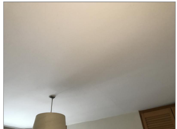
Photo - 81 Rear bedroom ceiling.
