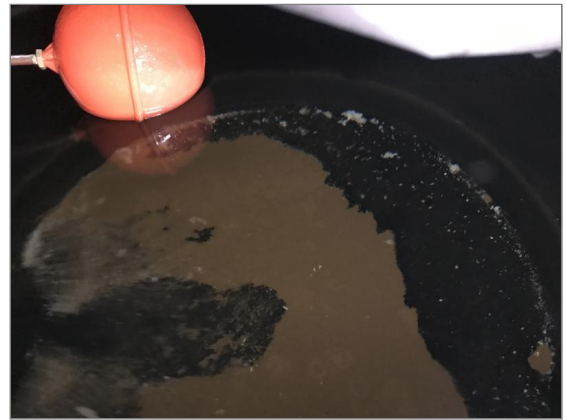
Photo - 168 Sediment build up in tank.
