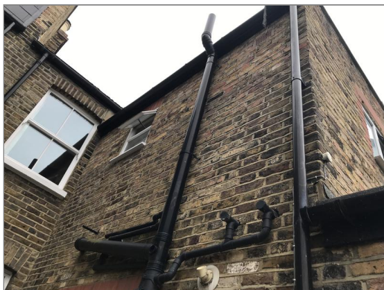
Photo - 178 uPVC soil stack at the rear of the property.
