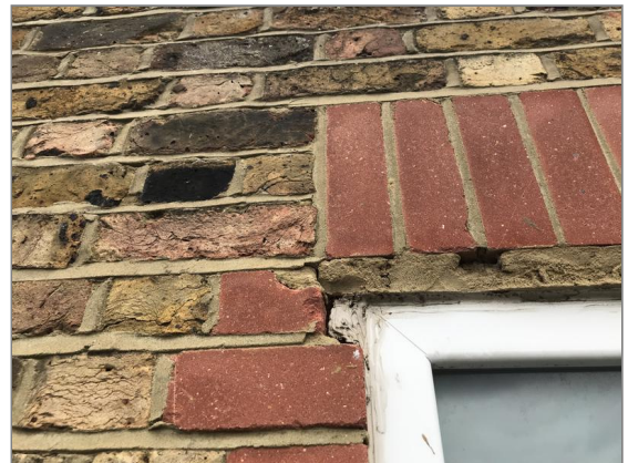
Photo - 35 Minor repair required to rear bathroom walls.
