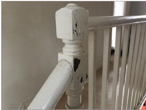
Photo - 153 Failure of decorations to stairs.
