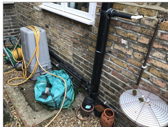
Photo - 179 uPVC soil stack and inspection chamber in the rear garden.
