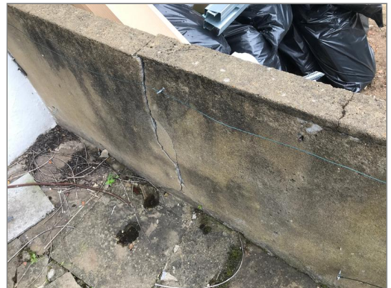
Photo - 185 Damage to front garden wall.
