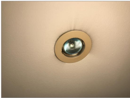
Photo - 165 Dated light fitting.
