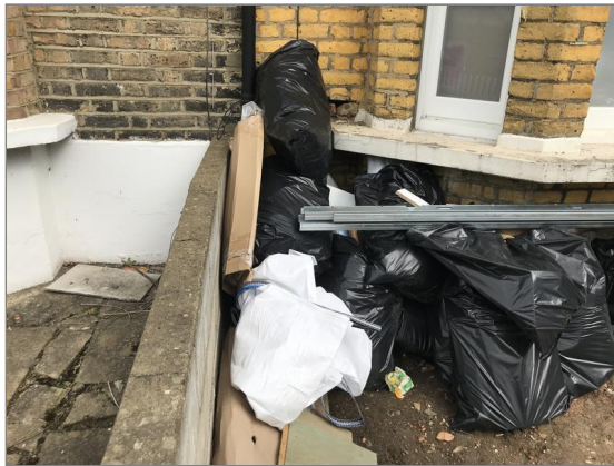
Photo - 22 Rainwater downpipe running into neighbouring garden.
