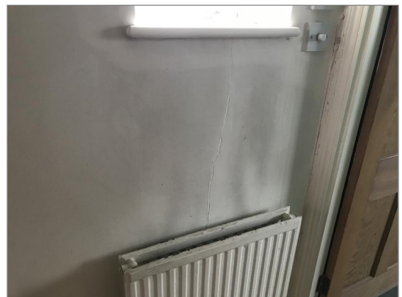
Photo - 116 Cracking to first floor landing walls.
