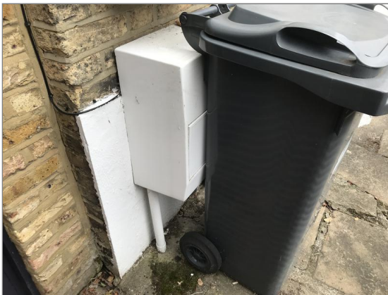
Photo - 166 Gas meter cabinet.
