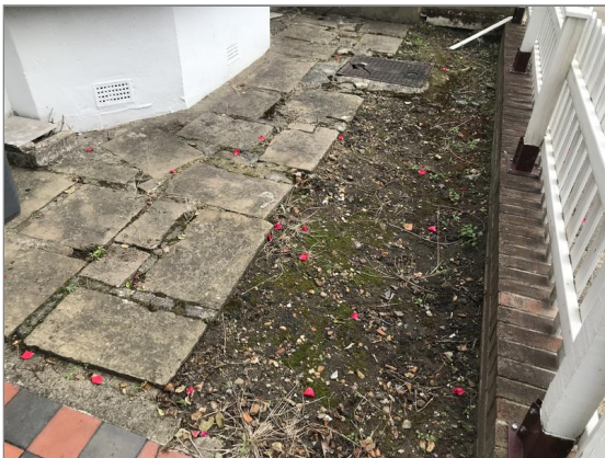
Photo - 184 Failure of paving in front garden.
