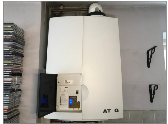
Photo - 171 Boiler in the kitchen.
