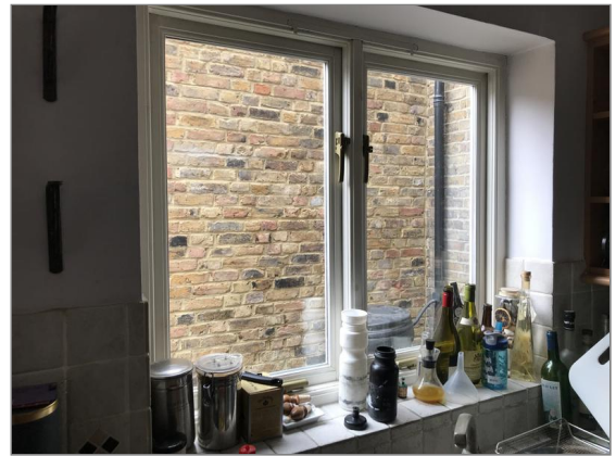
Photo - 58 Kitchen window.
