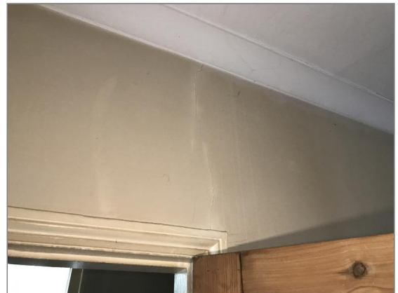
Photo - 114 Cracking above door leading to sitting area.
