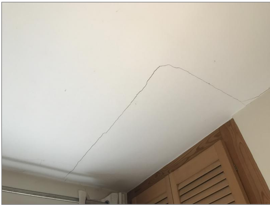
Photo - 82 Cracking to the bedroom ceiling.
