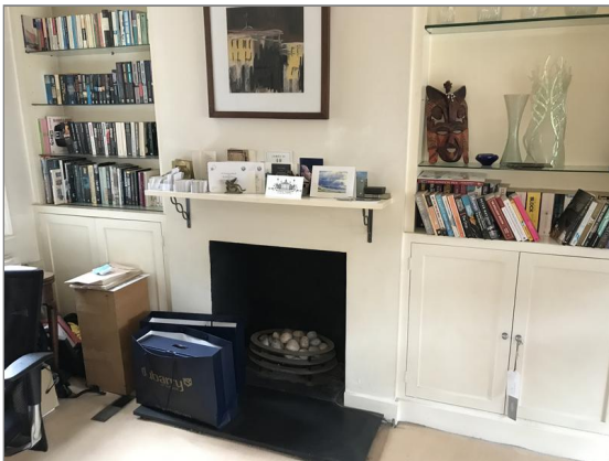
Photo - 143 Living area gas fire.
