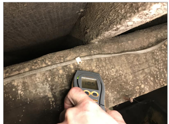
Photo - 79 Damage to roof timbers.
