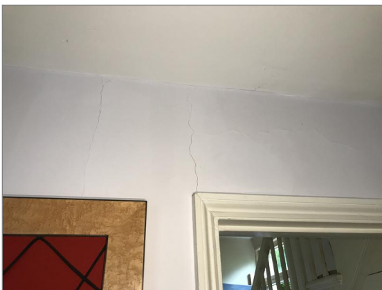
Photo - 103 Cracking to kitchen walls.
