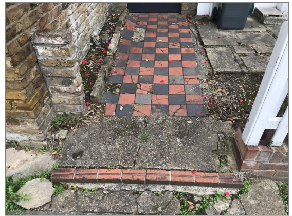
Photo - 183 Failure of paving in front garden.
