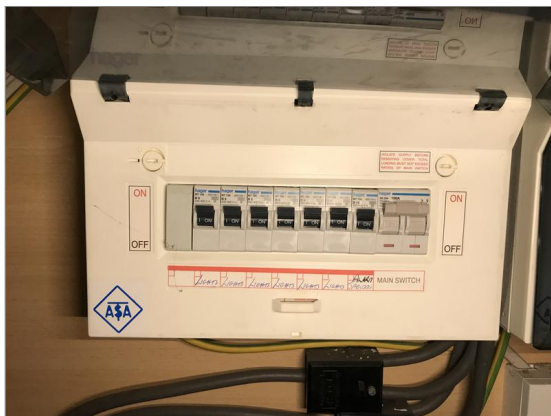
Photo - 163 Non RCD protected light circuits.
