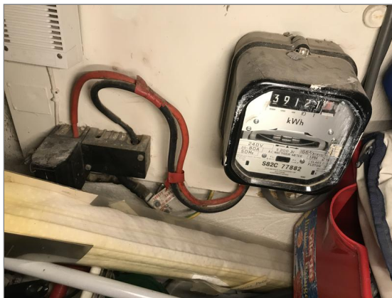
Photo - 161 Electricity meter.
