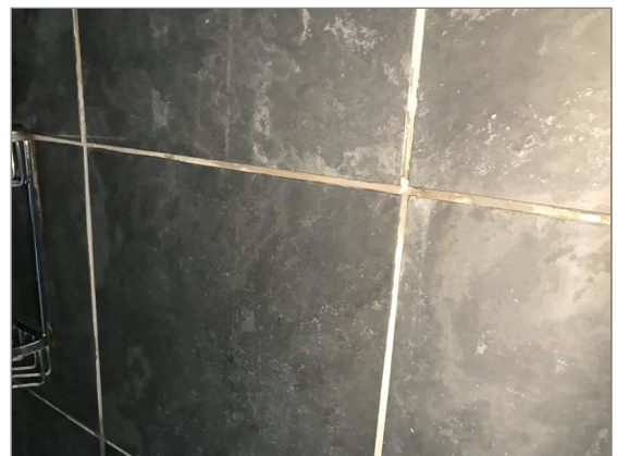
Photo - 122 Failure of tiling in shower enclosure.
