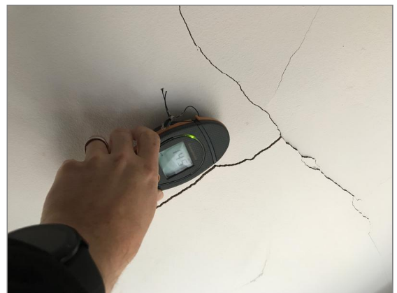
Photo - 93 Damage to kitchen ceiling.
