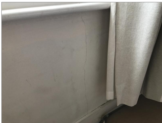
Photo - 127 Cracking to front bedroom walls.
