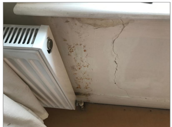
Photo - 128 Cracking to front bedroom walls.
