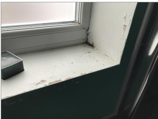
Photo - 121 Humidity damage to bathroom walls.
