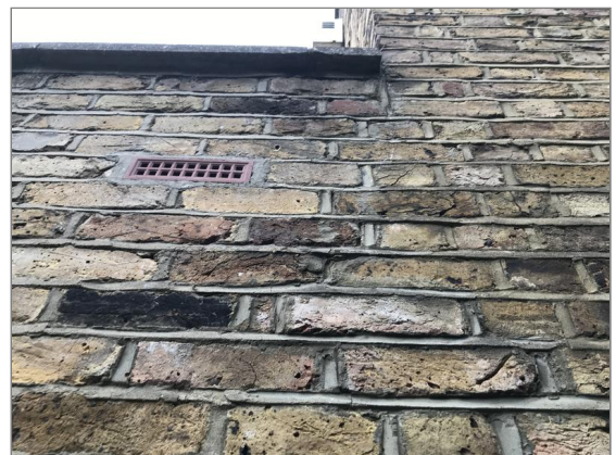
Photo - 37 Cracking at abutment of rear addition and original part of the property.
