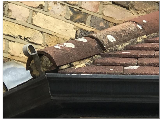
Photo - 10 Failure of mortar below ridge tiles.
