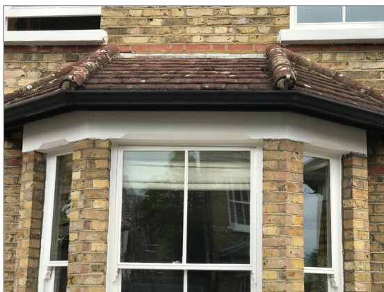
Photo - 30 Slight deflection of bay structure.
