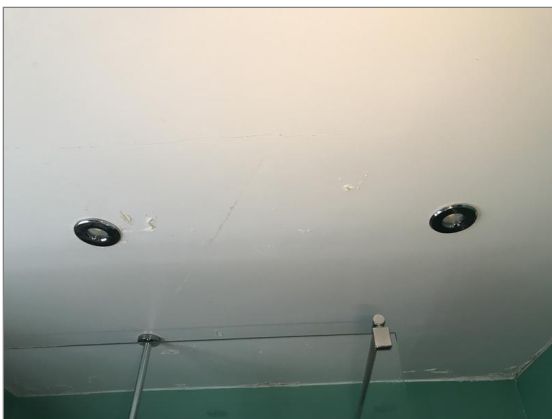
Photo - 86 Humidity damage to bathroom ceiling.
