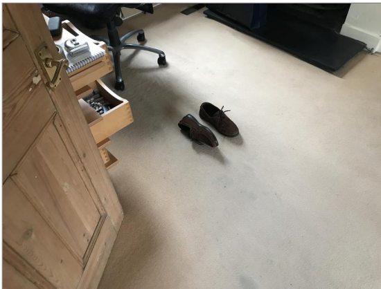
Photo - 137 Living carpet in tired condition.
