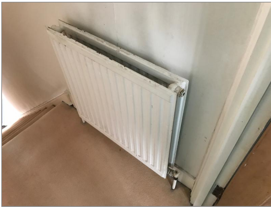
Photo - 170 Rust to radiator.
