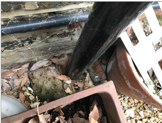
Photo - 26 Debris in middle gully.
