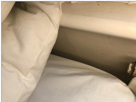
Photo - 131 Cracking to rear bedroom walls.
