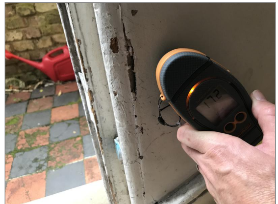
Photo - 108 Damp meter testing to entrance hallway walls.
