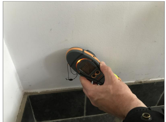
Photo - 96 Damp meter testing to dining area walls.
