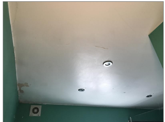
Photo - 85 Humidity damage to bathroom ceiling.
