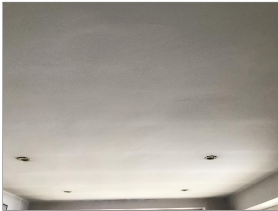
Photo - 94 Thermal shadowing to rear addition ceiling.
