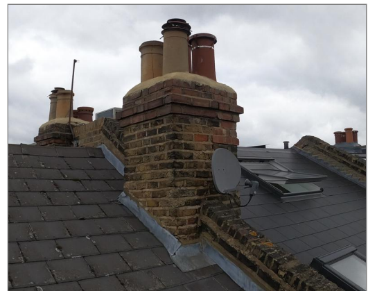
Photo - 7 Elevation view of front stack.
