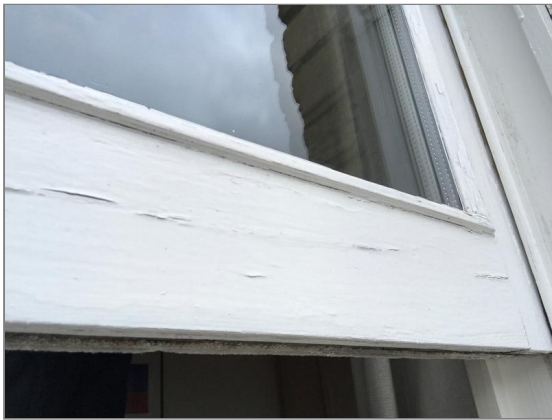
Photo - 45 Failure of decoration to front bedroom window.
