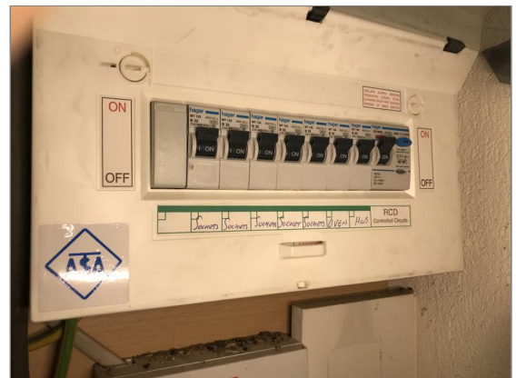
Photo - 164 RCD protected distribution board.
