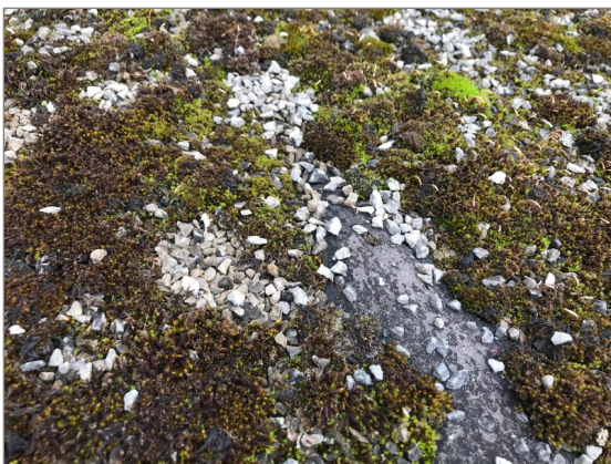
Photo - 19 Failure of felt to ground floor extension roof.
