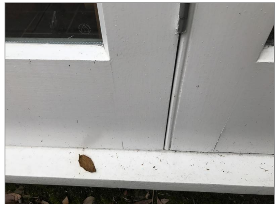
Photo - 67 Condition of folding doors.
