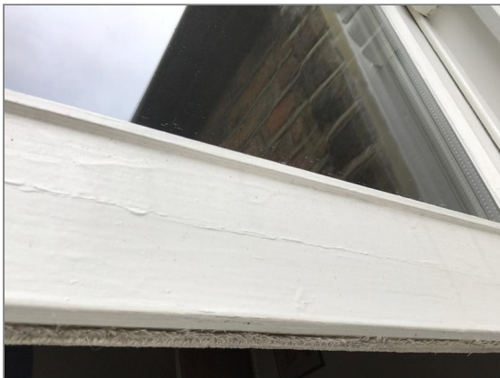
Photo - 47 Failure of decorations to rear bedroom window.
