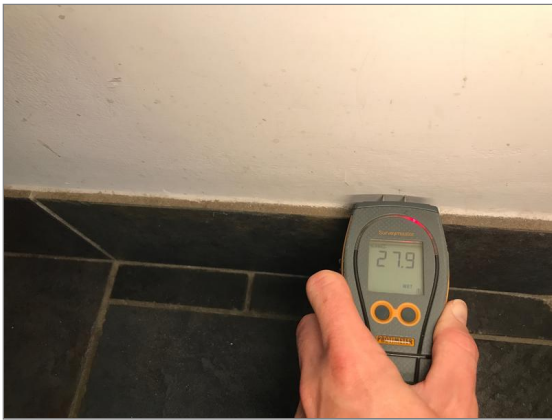
Photo - 105 Dampness to kitchen walls.
