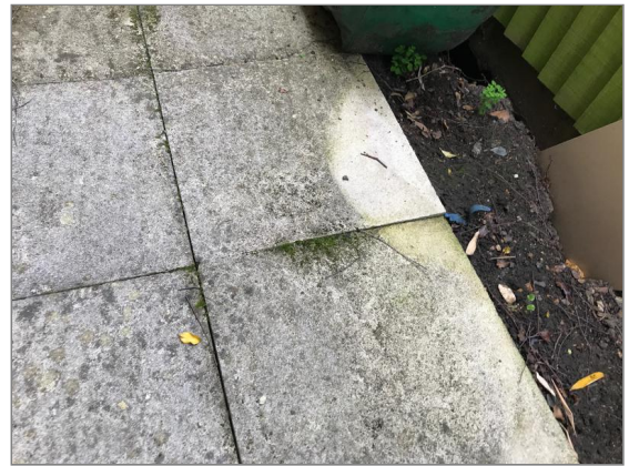
Photo - 189 Paving slabs require re-laying to the side of the property.
