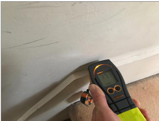
Photo - 107 Damp meter testing to entrance hallway walls.
