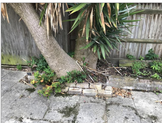
Photo - 192 Damage to wall in rear garden.
