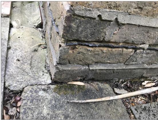
Photo - 38 Damp proof membrane to rear addition.
