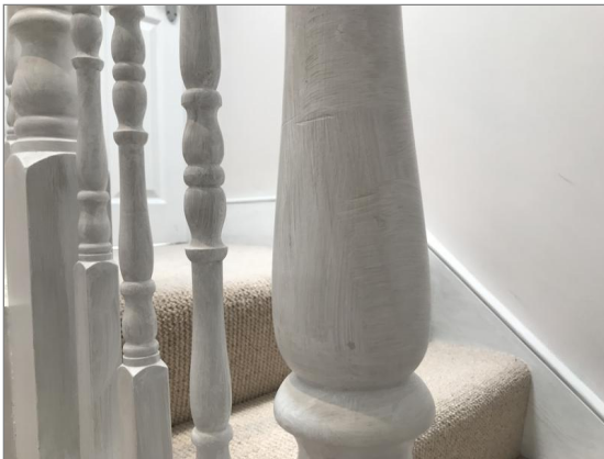
Photo - 185 Inexpert decorations to stairs
