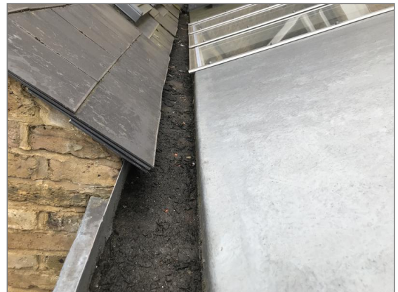
Photo - 30 Debris build up in valley gutter
