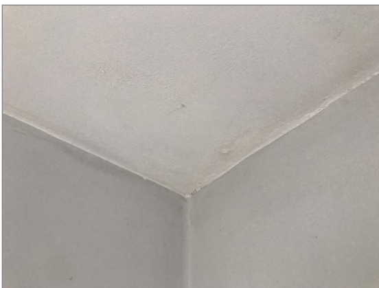
Photo - 96 Water damage to rear first floor bedroom ceiling
