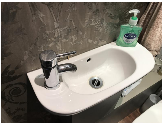
Photo - 124 Lack of splashback to WC walls
