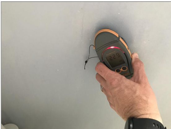
Photo - 146 Elevated damp meter readings to second floor bathroom walls
