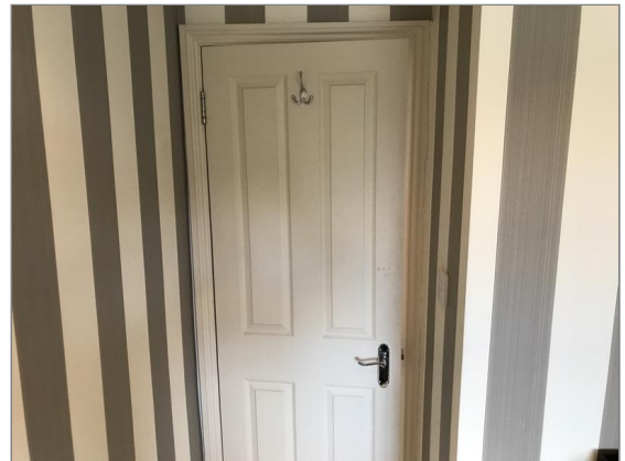
Photo - 186 Door binding upon frame to rear second floor bedroom
