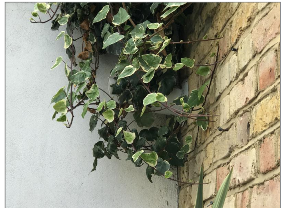
Photo - 173 Boiler flue obscured by plant growth
