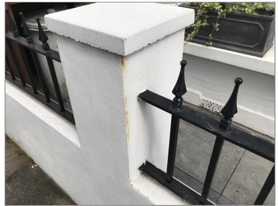
Photo - 224 Failure of decorations to front garden wall
