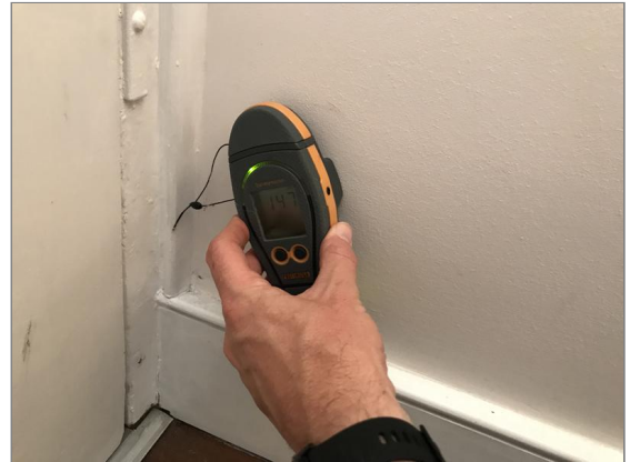
Photo - 105 Damp meter testing to entrance hallway walls
