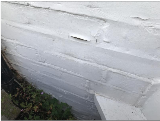
Photo - 34 Failure of decorations to front of property
