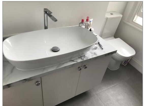
Photo - 193 Master en-suite fittings
