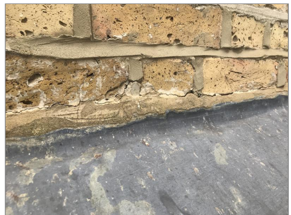
Photo - 22 Slight cracking to cement holding flashings of side addition roof in place
