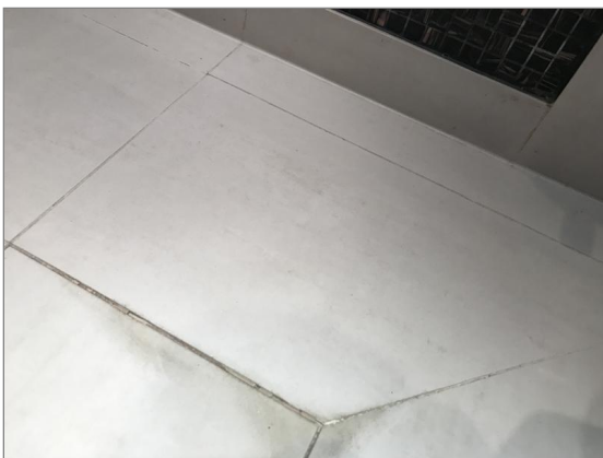
Photo - 160 Loose tiles to shower enclosure
