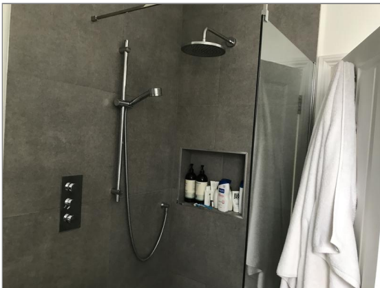
Photo - 196 Master en-suite fittings
