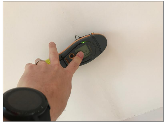
Photo - 93 Damp meter testing to area of cracking repair on first floor landing
