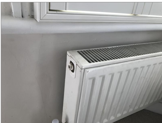
Photo - 136 Decorative damage below master bedroom windows
