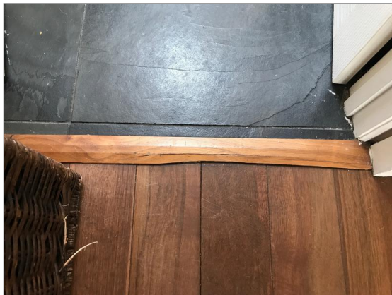
Photo - 164 Damaged threshold strip
