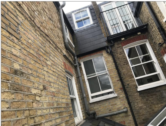
Photo - 218 Soil pipe at rear of property
