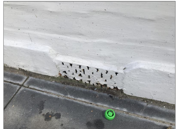
Photo - 33 Sub-floor vent in contact with ground
