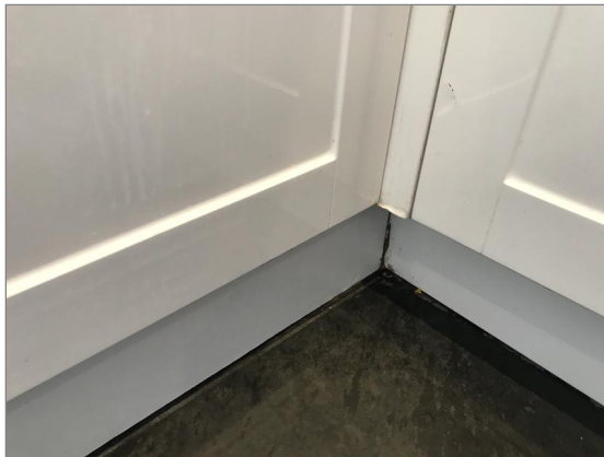
Photo - 182 Water damage to kitchen sink cupboard
