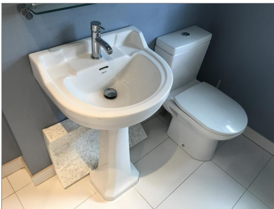
Photo - 190 Second floor bathroom fittings
