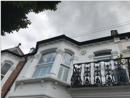
Photo - 23 Rainwater guttering at front of property
