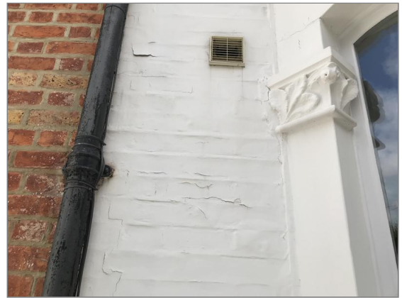
Photo - 35 Failure of decorations to front of property
