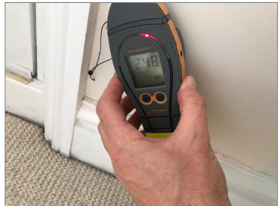
Photo - 135 Damp meter testing to master bedroom walls
