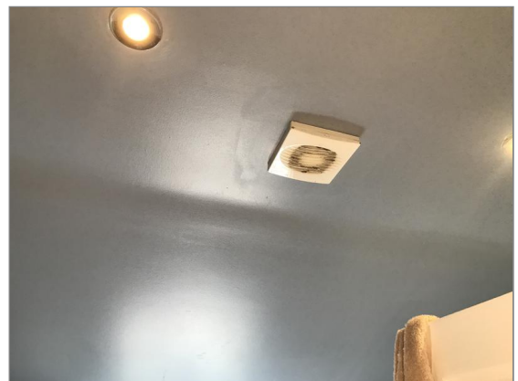
Photo - 85 Second floor bathroom ceiling
