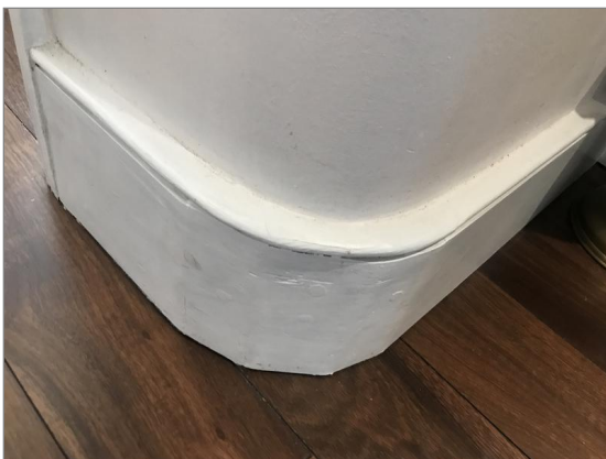
Photo - 189 Scuffing to skirtings at ground floor level
