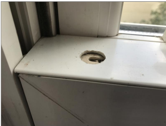
Photo - 54 Minor damage to rear first floor bedroom window
