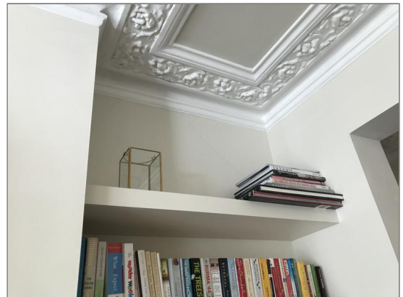
Photo - 111 Minor cracking to front sitting room walls
