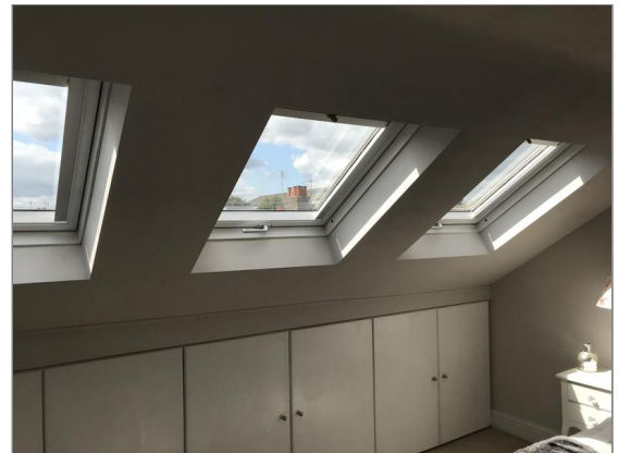
Photo - 77 Deflection of front pitched roof structure
