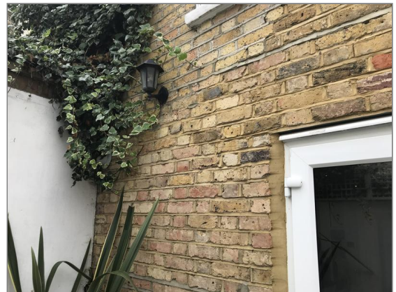
Photo - 43 Hard paving directly abutting external walls
