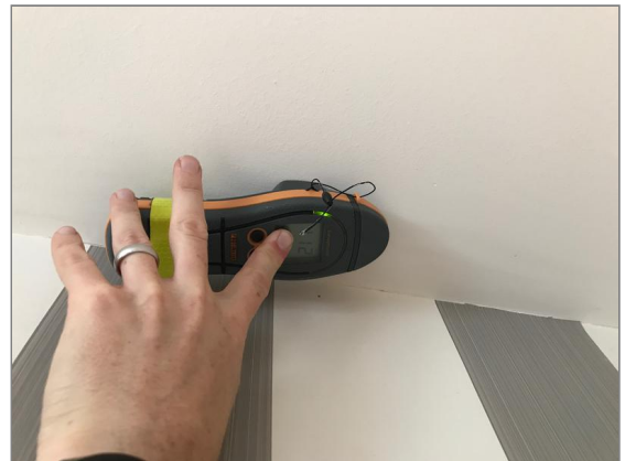
Photo - 89 Damp meter testing to area of water staining
