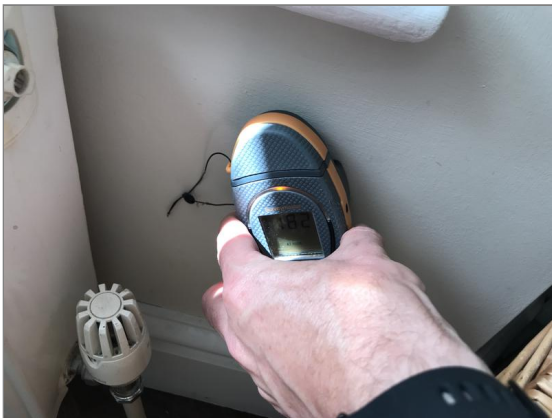
Photo - 110 Damp meter testing to front sitting room walls
