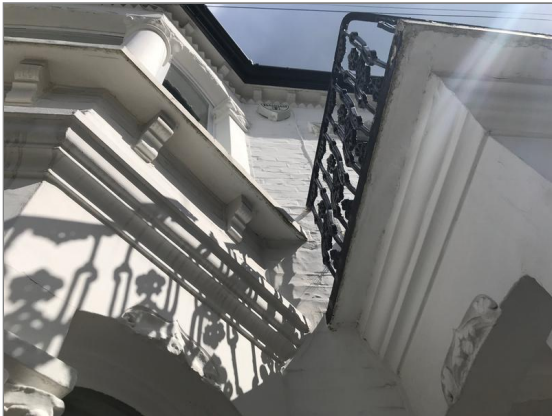
Photo - 36 Failure of decorations to front of property
