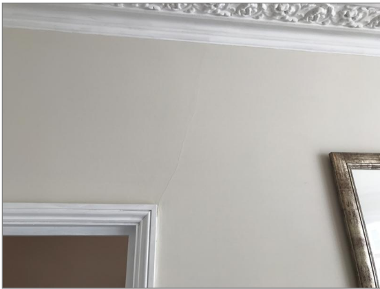
Photo - 108 Cracking to front sitting room walls
