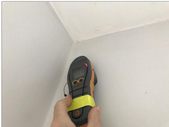
Photo - 126 Dampness to rear first floor bedroom walls
