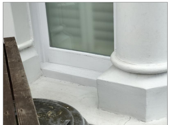
Photo - 57 Slight failure of decorations to front sitting room windows
