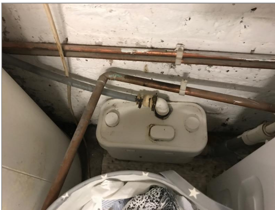
Photo - 220 Saniflo unit in basement
