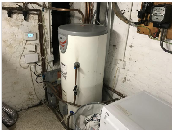
Photo - 217 Hot water cylinder in basement
