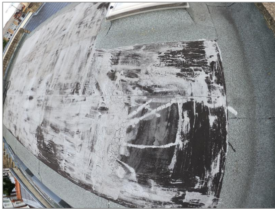
Photo - 17 Waterproof paint used to prolong the life of flat mansard roof
