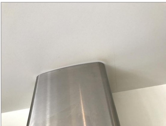
Photo - 102 Kitchen ceiling
