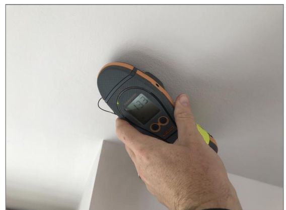
Photo - 79 Damp meter testing to second floor bedroom ceiling
