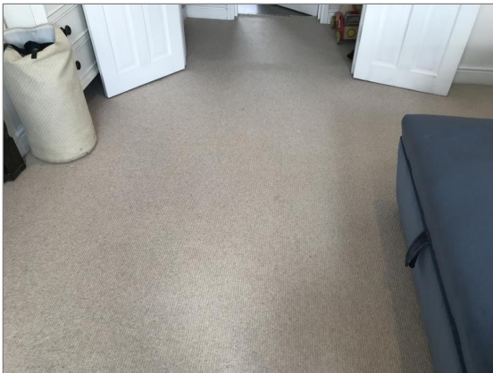
Photo - 156 Unevenness to master bedroom floor
