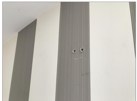
Photo - 143 Mechanical damage to rear second floor bedroom walls
