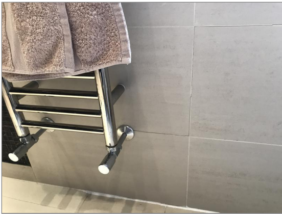
Photo - 132 Cracking to bathroom tiling
