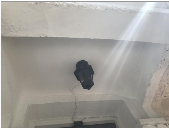
Photo - 70 Slight water damage to porch soffit
