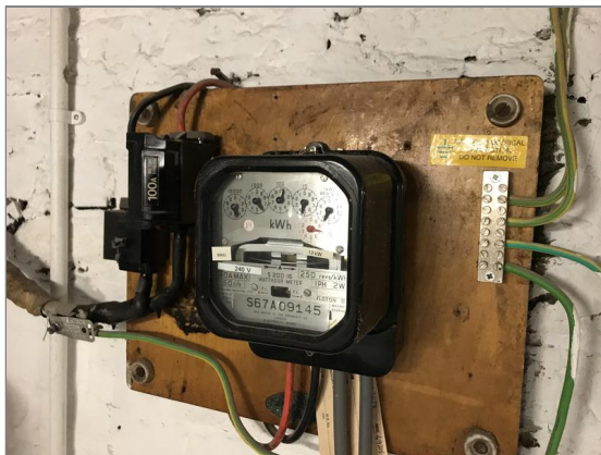
Photo - 205 Incoming main and meter
