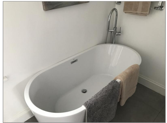
Photo - 195 Master en-suite fittings
