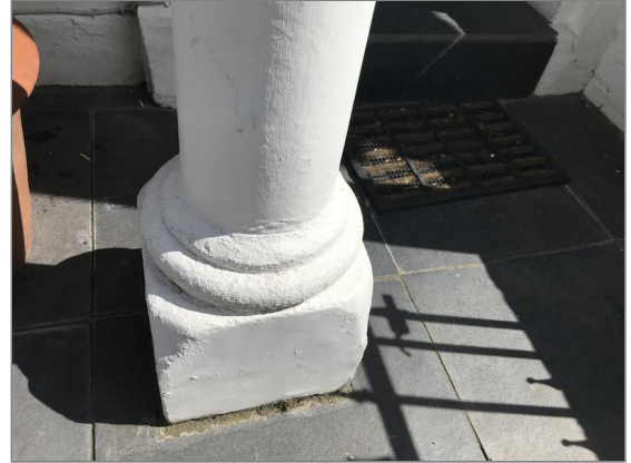
Photo - 69 Failure of decorations to porch
