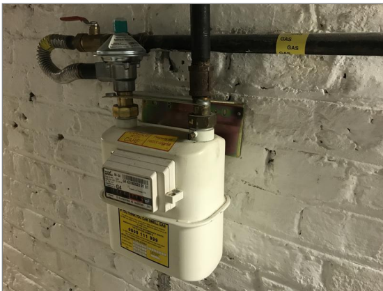
Photo - 208 Gas meter
