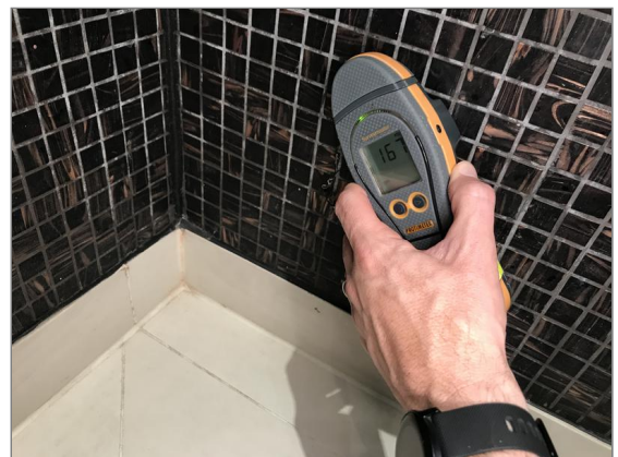
Photo - 131 Damp meter testing to tiling
