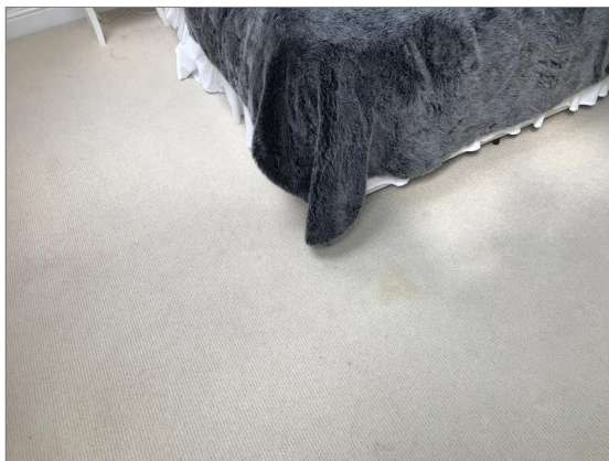
Photo - 152 Staining to larger second floor bedroom carpet
