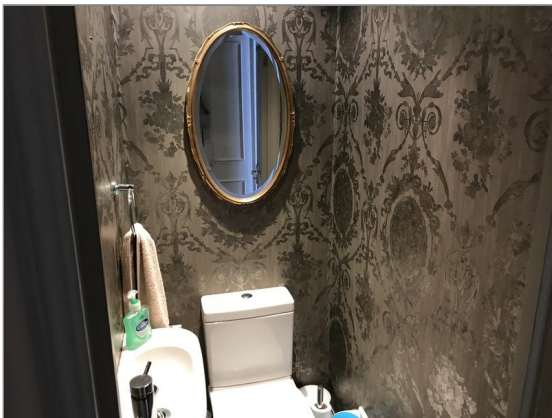
Photo - 122 Downstairs WC walls
