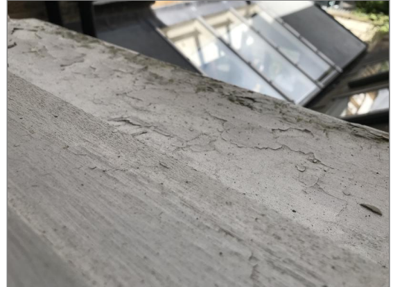
Photo - 74 Decorative condition of window sills
