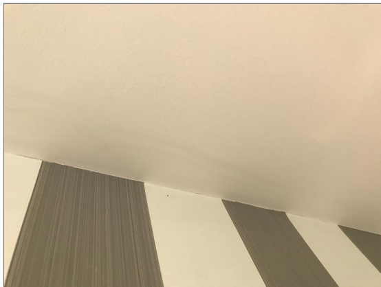
Photo - 88 Water staining to rear second floor bedroom ceiling
