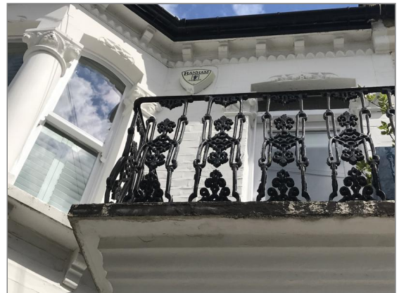
Photo - 71 Damage to metal railings surrounding porch
