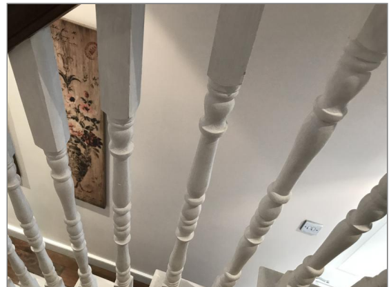
Photo - 188 Inexpert decorations to stairs
