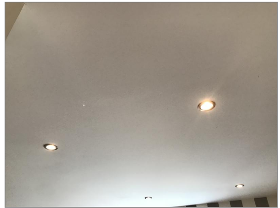
Photo - 87 Rear second floor bedroom ceiling
