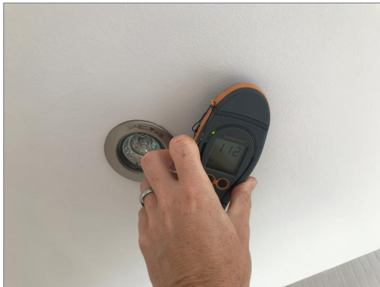
Photo - 80 Damp meter testing to second floor bedroom ceiling
