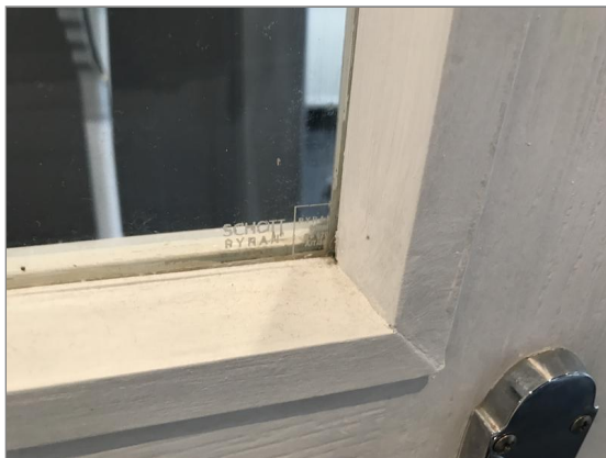
Photo - 4 Fire rated glass fitted to door
