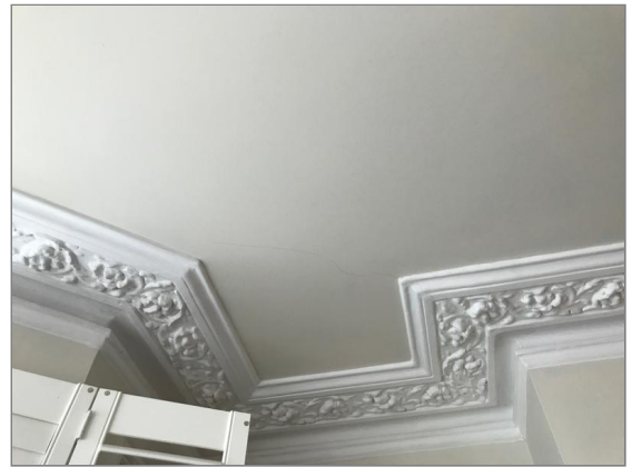
Photo - 99 Hairline cracking to front sitting room ceiling
