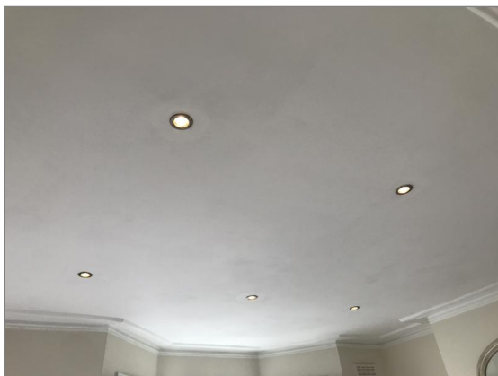
Photo - 90 First floor master bedroom ceiling
