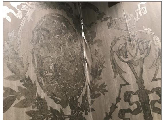
Photo - 123 Failure of decorative lining paper to WC walls
