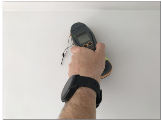
Photo - 167 Damp meter testing to chimney breast at second floor level
