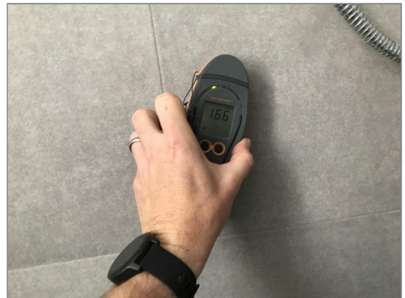
Photo - 141 Damp meter testing to tiling
