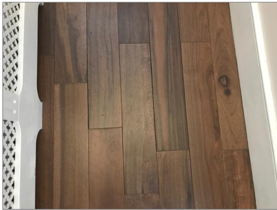
Photo - 162 Joints opening up between timber boards to entrance hallway
