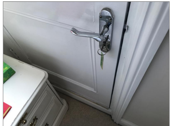
Photo - 65 Master bedroom door requiring adjustment
