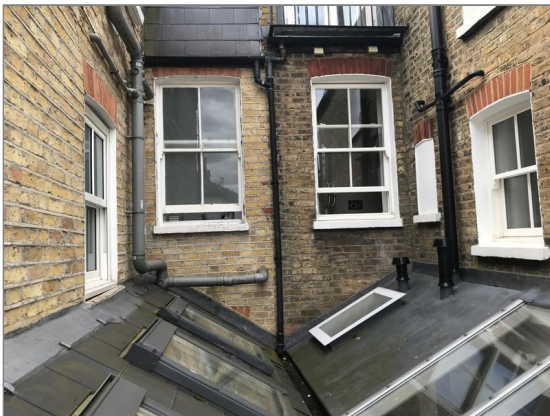
Photo - 29 Downpipe discharging into valley gutter at rear of property
