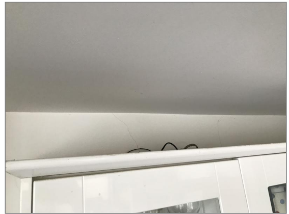
Photo - 121 Slight cracking to kitchen walls
