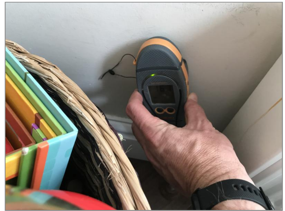
Photo - 109 Damp meter testing to front sitting room walls
