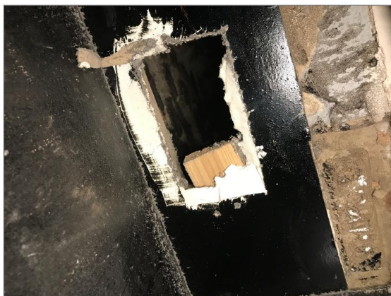
Photo - 170 Ventilation to fireplace in master bedroom
