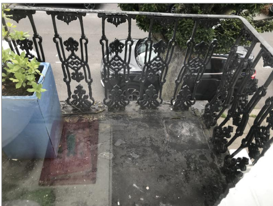
Photo - 72 Failure of waterproofing to porch soffit
