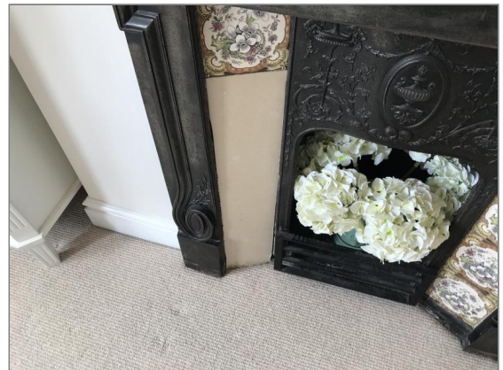
Photo - 169 Missing tiles to side of chimney breast
